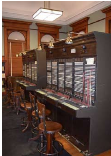
Vintage switchboards were brought in to complete the transformation of the Society's headquarters into the Cape Cod Bell Telephone Company, circa 1952.
